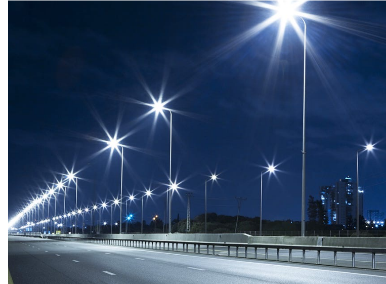
Poorly designed LED streetlights
